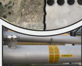
gas cooler, gas pipings
