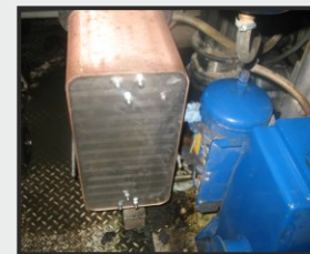
plate heat exchanger
