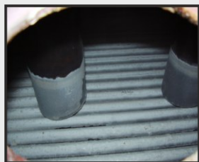
boiler fume gas side and water, steam side
